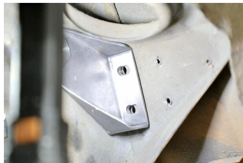
Figure 66 - Drill Floor Pan Holes
